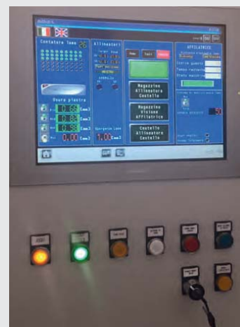
CONTROL PANEL WITH REMOTE ASSISTANCE
